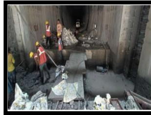
HM work Site clearance and cleaning at MIG and BMIG of Intake -1
