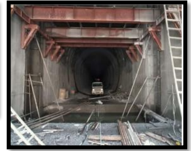
HM Work Site clearance and cleaning at MIG and BMIG of Intake -2
