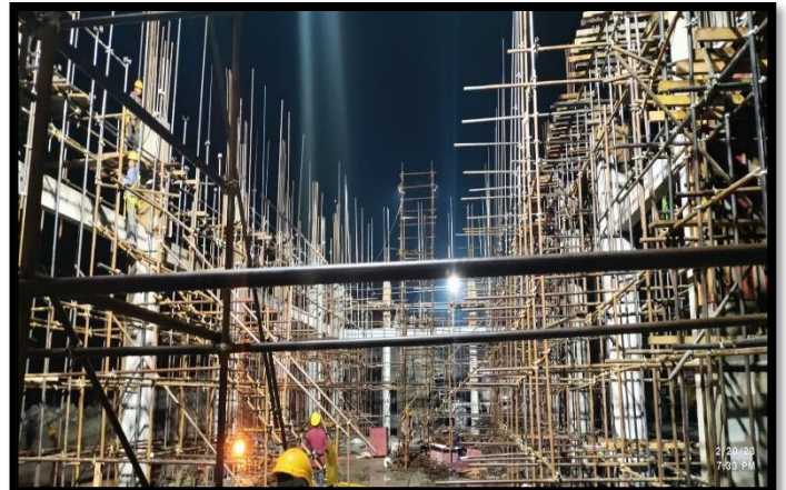
GIS Raft A Portion
